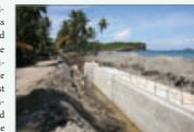
This sea wall is being built in St. Patrick, Grenada, after tons of sand was stolen from the beach, opening the area to erosion.
